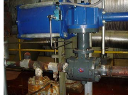
The MOGAS SC-3PC was chosen to replace a leaking globe type valve on a HP turbine bypass line. The isolation valve must seal during online operation to avoid leaking boiler feedwater through the control valve.
