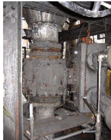
Shown above is the bottom, 16-inch lockhopper valve that endured several years of arduous service, cycling every 15 minutes and discharging erosive slurry.
