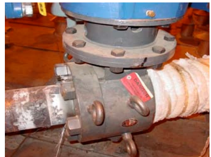
The C-Series valve was chosen for our customer's Boiler Purge System because of the rapid operation available with quick, quarter-turn rotation and absolute shut-off. These photos were taken during a routine maintenance shutdown with part of the insulation removed.
