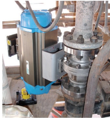
This MOGAS valve – with a sturdy mounting bracket, spring-loaded packing along with proper stem bushing alignment – provided a record 25,000 cycles, greatly improving runtime.
