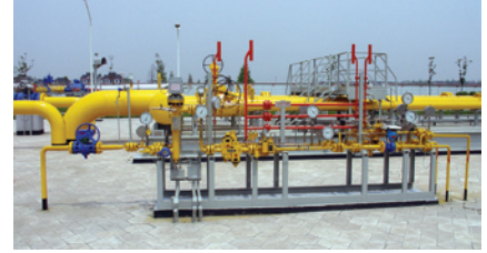
In this compressor station located in Beijing, China, these FlexStream valves are precisely controlling Pressure Reduction to safeguard the local gas distribution networks.
