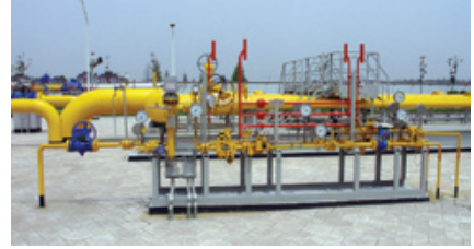
In this compressor station located in Beijing, China, these FlexStream valves are precisely controlling Pressure Reduction to safeguard the local gas distribution networks.
